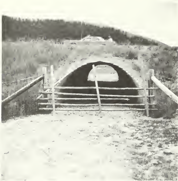
EAST ENTRANCE; water and mud backs up beyond entrance.
